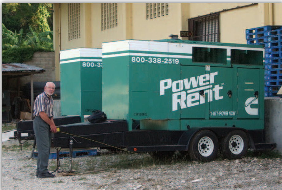
Generator units purchased for use in Haiti
