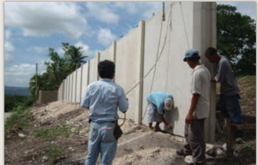
Workers construct the first 150 feet of the new security wall at La Loma Luz Hospital in Belize. It takes more than four weeks of construction per 150 feet of fence. ▲
