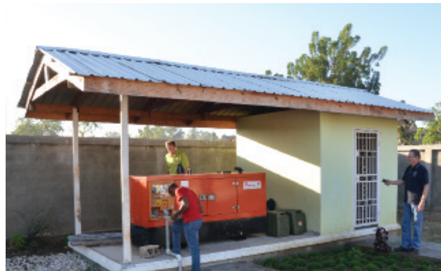
Ken Breyer (center, top), facility construction and maintenance for AHI-Global, and Jerry Daly (right), logistical support for AHI-Global, inspect a generator at Hopital Adventiste d’Haiti.
